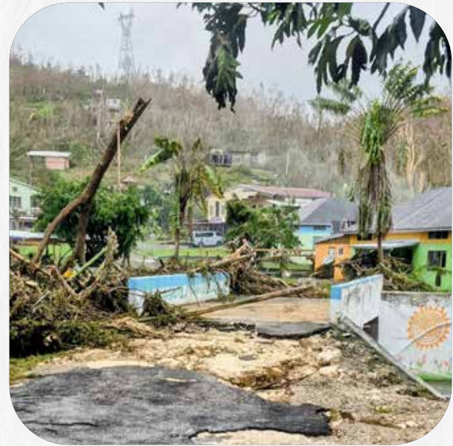
Hurricane damage to the Mustard Seed Communities home for the disabled in Montego Bay
